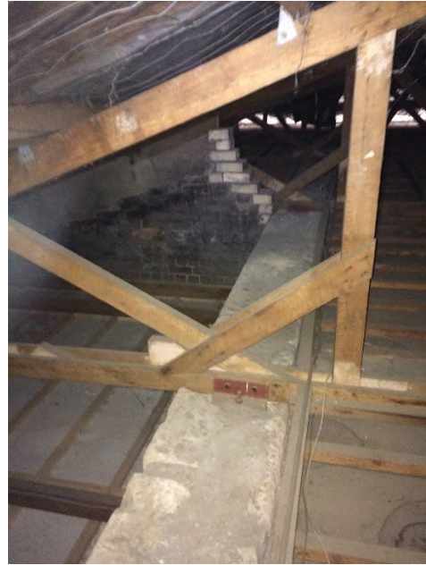
Figure 79. 1960s timber roof and ceiling framing to main building. Figure 80. Inside roof – tops of stone and brick walls.
