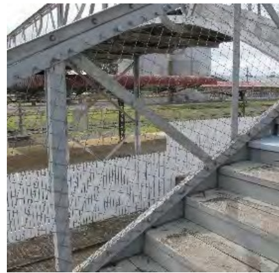
Figure 101. Non-original timber and chain wire inserts.
